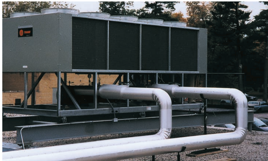
This air-cooled chiller and related piping serve a hospital's surgery and patient rooms. Planned maintenance and inspections ensure the integrity of this system.
