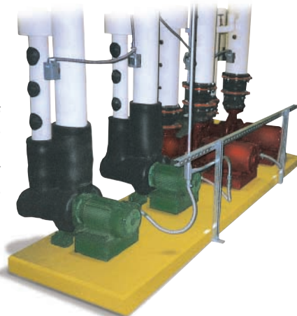
These circulating pumps, used in conjunction with chiller systems like the one at right, were designed and installed by August Winter & Sons.
